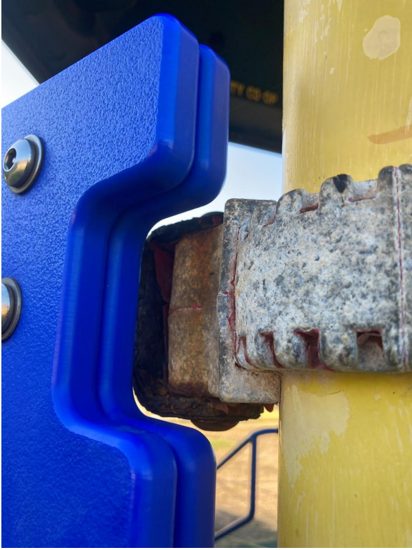
Pictured: Current structure in deteriorated condition.
